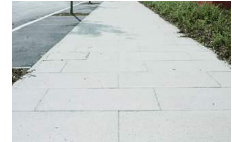
PAVING TYPE C: Granite aggregate concrete slabs, 600x 600 x 50mm - Charcon 'Appalachian' Black Fleck ground chamferless
